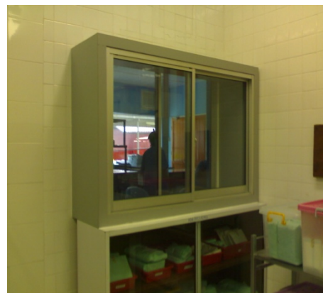
Air lock at distribution area
