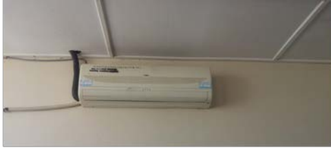
Picture 2. One air-conditioner in autopsy room.
