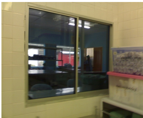
No air lock at distribution area
