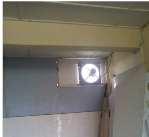
Picture 4. Exhaust fan which is located in autopsy room.
